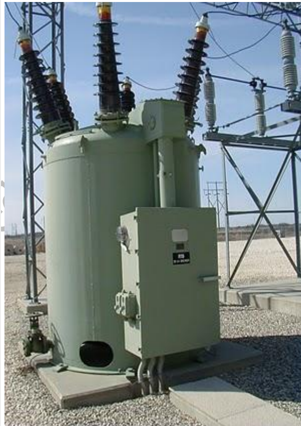
( b ) 66 KV circuit breaker
