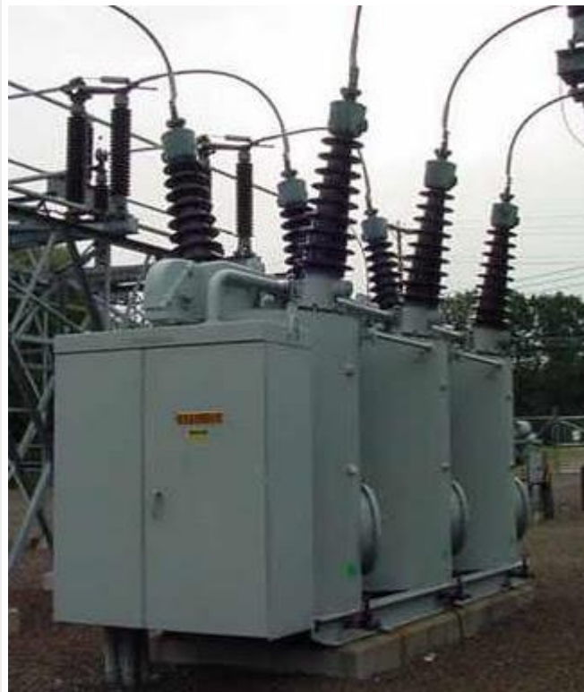
( a ) 115 KV circuit breaker
